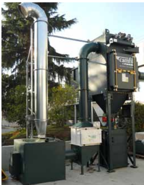
The design of the dust collector system was developed in cooperation with the customer's engineering and maintenance team in order to achieve the best performance in terms of ergonomics and safety.
